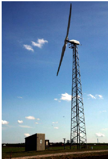
Figure 4: Gaia wind turbine
